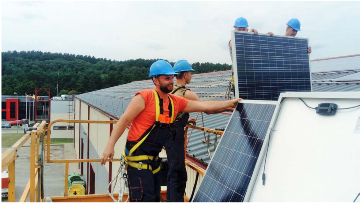
Picture 7. 9 Solar pannels beeing installed on a municipal building of Vilnius city maintenance institution „Grinda“.
