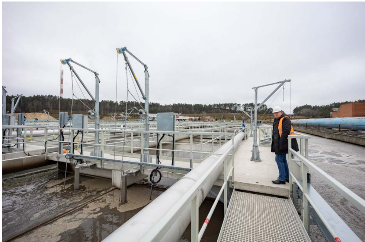
Picture 2. 2 Wastewater being cleaned in Vilnius wastewater treatment plant.
